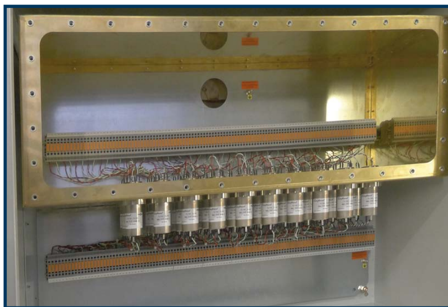
Inside of AAA cabinet
