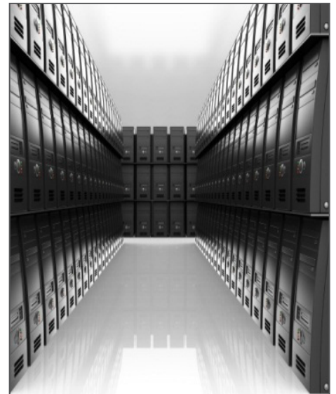
Servers at a Land-Based Military Communications Processing Center
